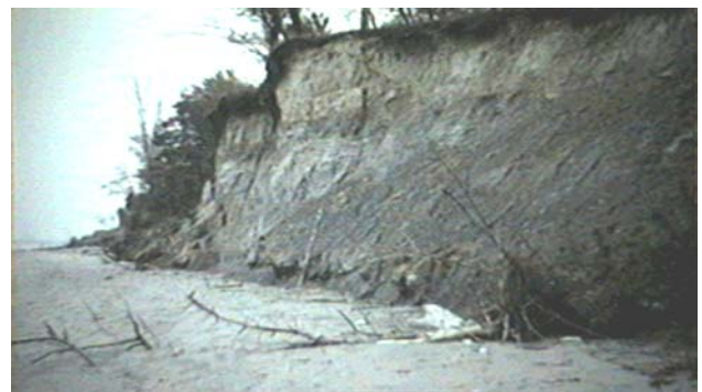
Figure 6: Failure of the overhangs and subsequent removal of talus material by wave activity maintained a near vertical profile at Site 1.
