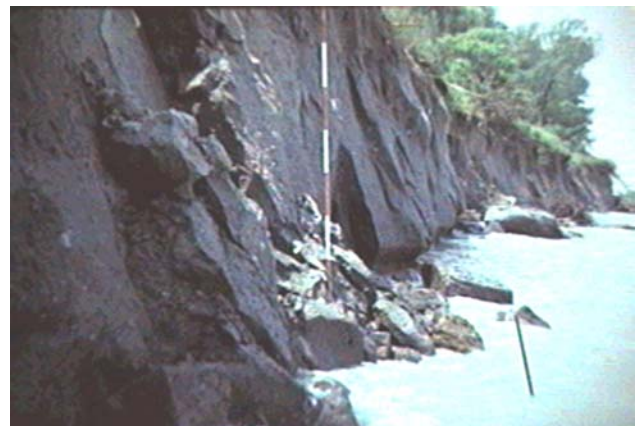
Figure 7: Notch development and subsequent plane failure at Site 2.
